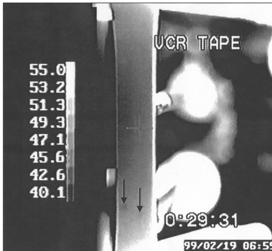
Figure 6 Debonding and spallation are visible with the VCR image, but the resolution and imaging frequency are relatively limited.
